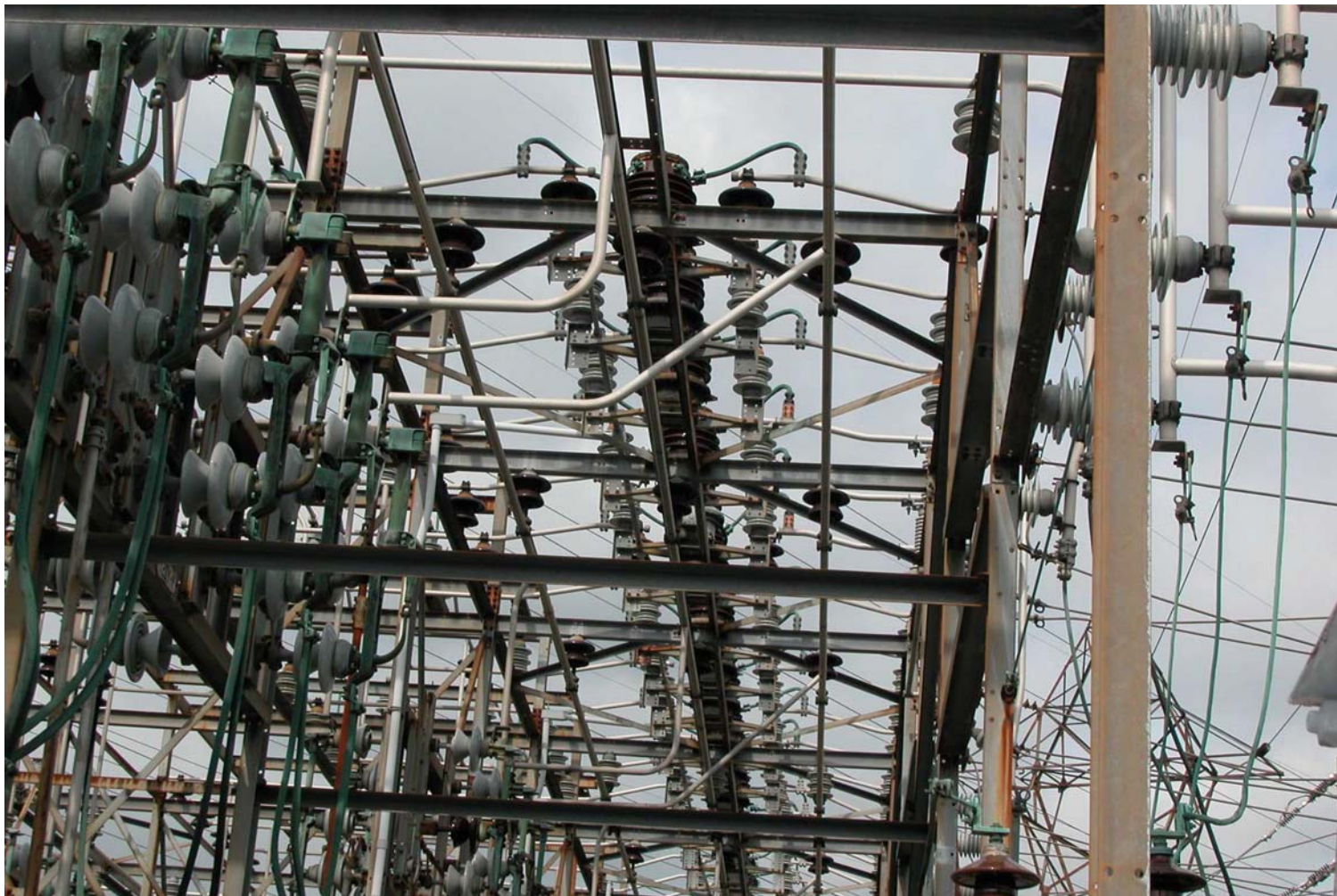
Leaside TS outdoor switchgear showing CTs
