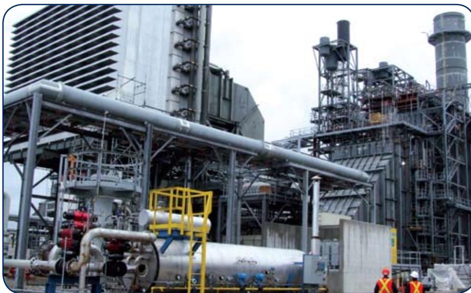
One of two natural gas-fired combustion turbines will generate up to 584 megawatts of electricity when commissioned in late fall.
